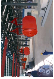
拥有16套专利地下电炉 16 Underground Patented Electric Furnace
